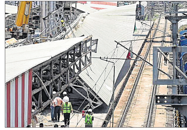
The portion of a tin shed that collapsed at Charbagh railway station in Lucknow on Friday.
